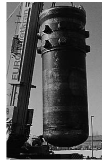
The pressure vessel, which weighs 250 tonnes, being lowered into position at the Paks training centre.
